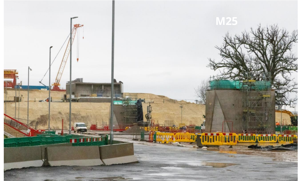
Construction of viaduct piers will continue in Bucks between the Hertfordshire border and the Colne River
