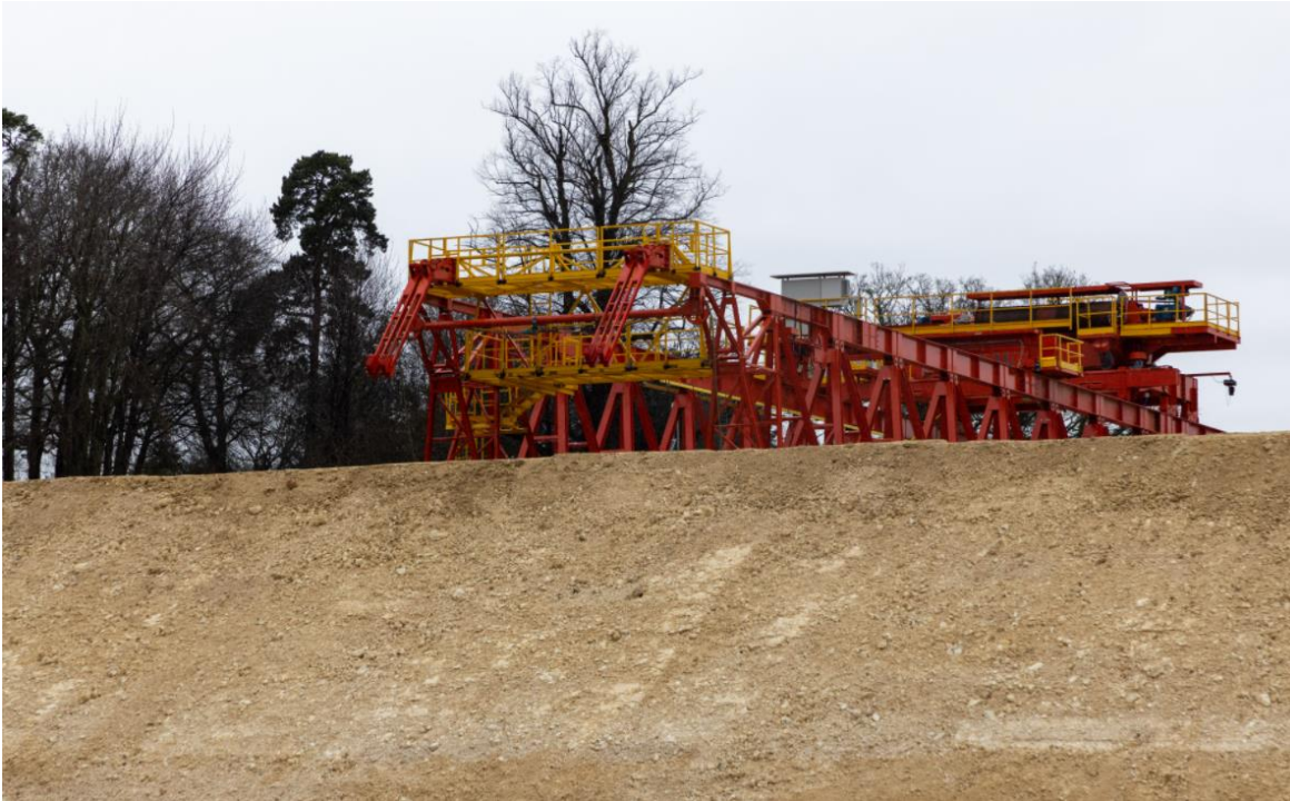
Viaduct deck gantry launches in Bucks, May 2022 and will lay deck as far as Denham Water-ski Club
